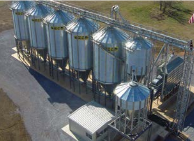
Installation of Grain Pump Loop System with a wet bin and dryer application.
